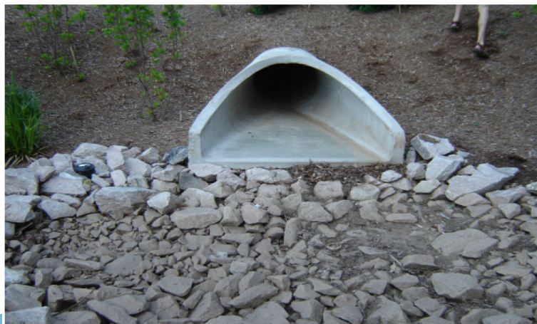
Figure 46: Rip-rap forebay (NCDENR 2007)
