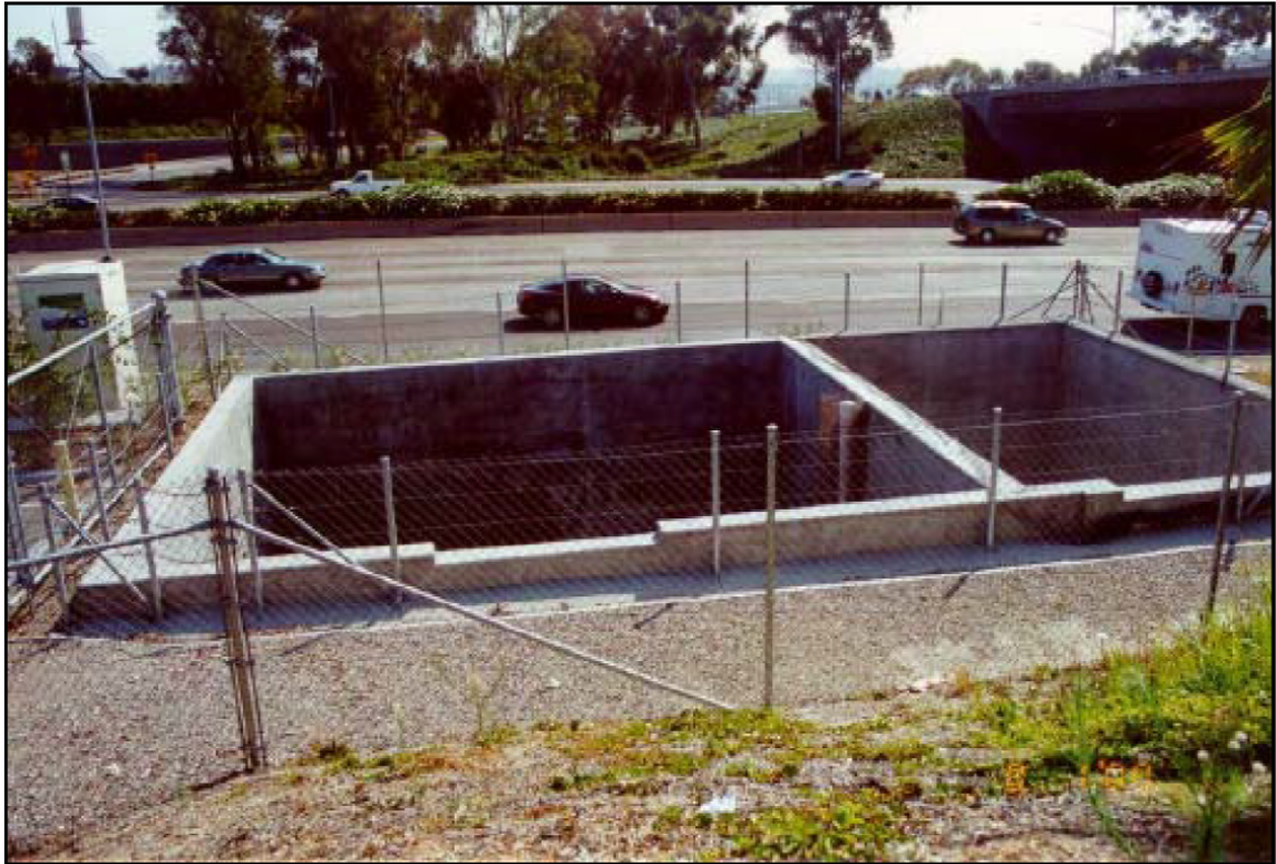
Figure 7: Sand filter for treatment of highway runoff (CalTrans 2004)
